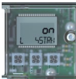
Maintenance Alarm set to be signaled
